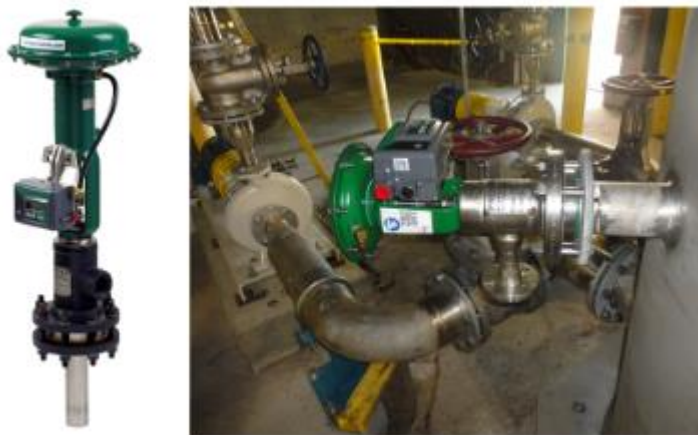
Fig. 2 - Example of Radial Multi-port Jet Diffuser Design mounted on a Hot Water Tank
